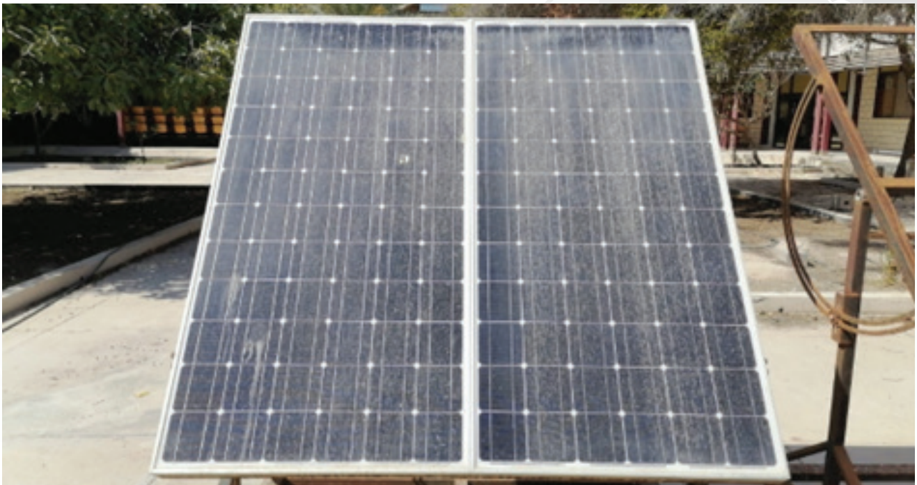
Dusty photovoltaic panel on the right, very dusty photovoltaic panel on the left
