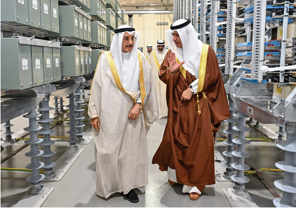
His Excellency Shaikh Khalid bin Abdulla Al Khalifa, Deputy Prime Minister, listens to an explanation from His Excellency Engineer Kamal bin Ahmed Mohammed, President of the Electricity and Water Authority (EWA), during a tour of Riffa offset station Interactive ability.
